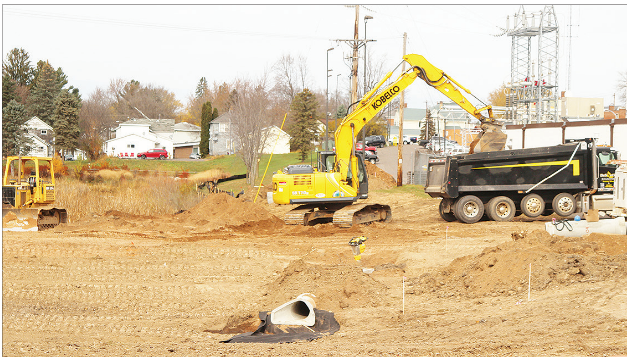
Work is well underway on the South East Storm Water Pond on the "Library Lake" portion of Beaver Dam Lake. This phase of the project will involve connecting 3 storm water drains from the City parking lot and several businesses along the alley to a new storm water pond. The pond will be the first of three treatment facilities to be located in the area where three houses were removed.
