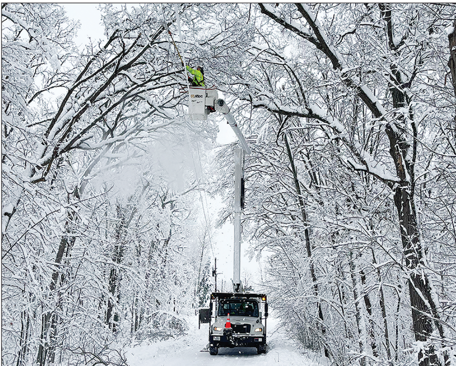
A Barron Electric crew member works to restore power after last week's storm cause widespread power outages.
